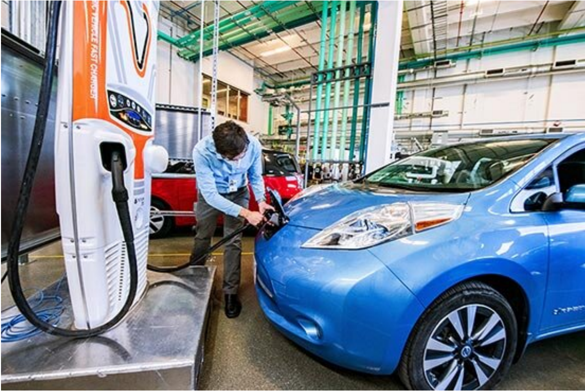
The Optimization and Control Lab's Electric Vehicle Grid Integration bays allow researchers to determine how advanced high power chargers can be added safely and effectively to the grid, with the potential to explore how to combine buildings and EV charging. Credit: Dennis Schroeder, NREL
