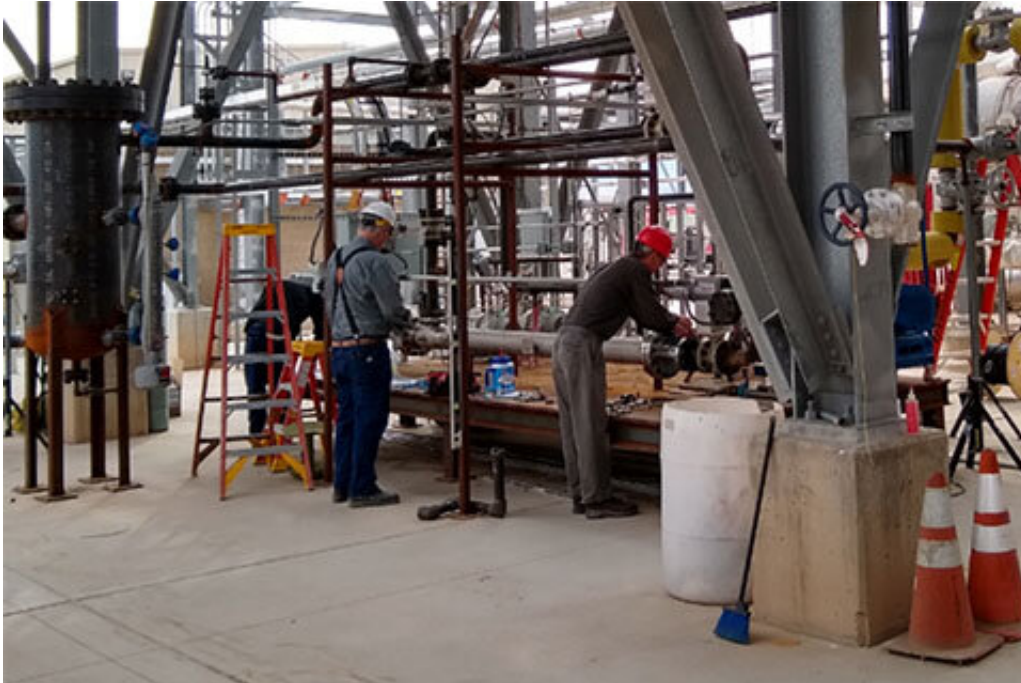
Installation of the integrated hydrogen sensor/separator module at Nevada Solar One. Credit: Koenraad Beckers, NREL
