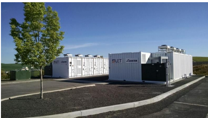
Vanadium redox storage system. Credit: Wikimedia
