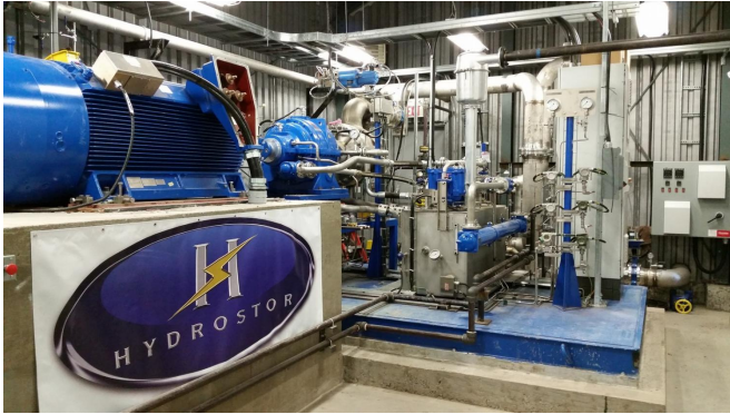
Hydrostor Advanced Compressed Air Energy Storage (A-CAES) demonstration facility, Toronto, Ontario. Credit: CNW Group/Hydrostor Inc.
