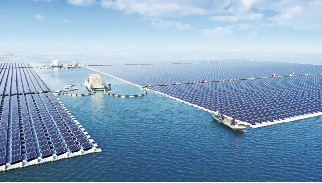
40MW Floating PV Power Plant. Credit: Sungrow
