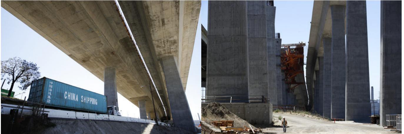
In this July 2, 2018, photo, a truck carrying a cargo container drives under the Gerald Desmond Bridge under construction in Long Beach, Calif. The new Gerald Desmond Bridge at the nation's second-busiest port isn't just a crucial route for cargo trucks and Southern California commuters - it's a concrete-and-steel science experiment for engineers and seismologists. It's slated to open next year. (AP Photo/Jae C. Hong)
