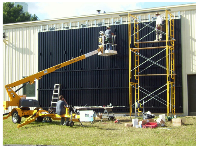
The installation of a solar wall at Wicked Joe's roastery in Maine. Credit: NASA
