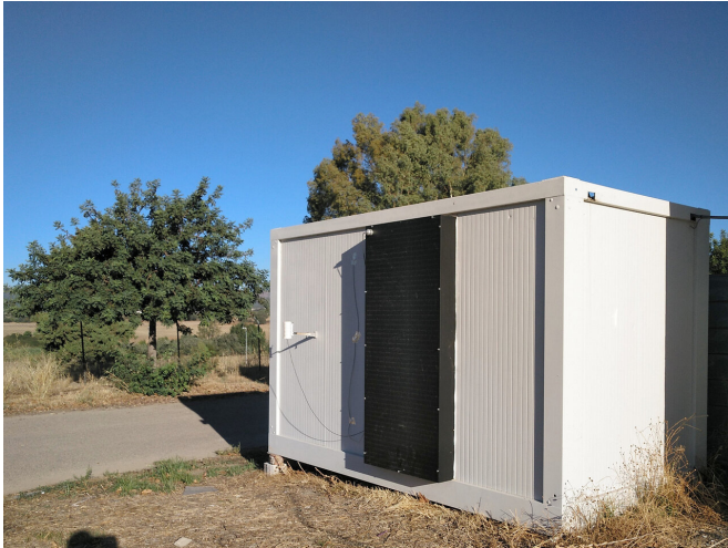
The device installed by the research team. Credit: University of Córdoba
