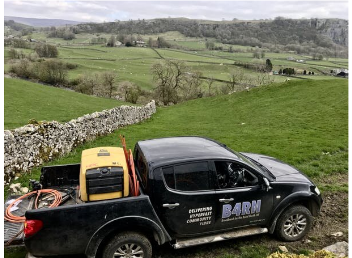
B4RN vehicle parked in a field in rural northwest England during a fibre installation. Credit: Kira Allmann, 2019, Author provided
