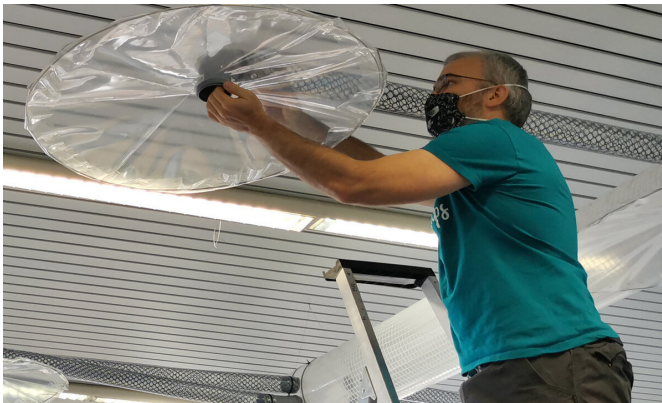
A simple exhaust air system for classrooms: Thomas Klimach assembles one of the hoods that will collect the warm air exhaled by students above a desk and direct it into the exhaust air duct. Also present: Roland Wollowski, Headmaster of IGS Mainz-Bretzenheim. Credit: Elena Klimach
