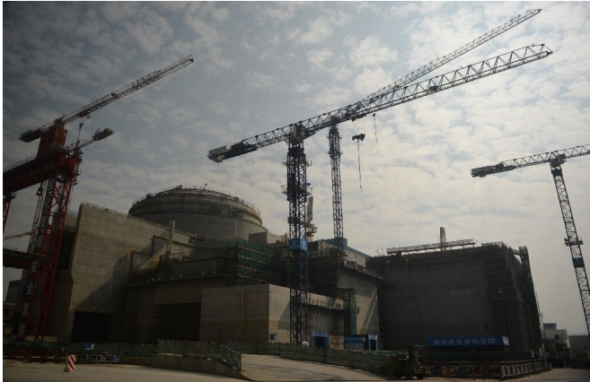
A years-long Chinese-French project, the Taishan nuclear power plant opened in 2018.
