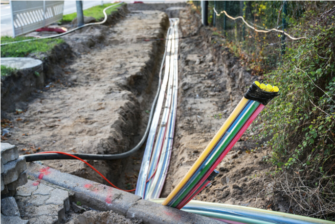
Fiber optic cables laid in a trench, to supply high-speed internet. Credit: University of Pennsylvania
