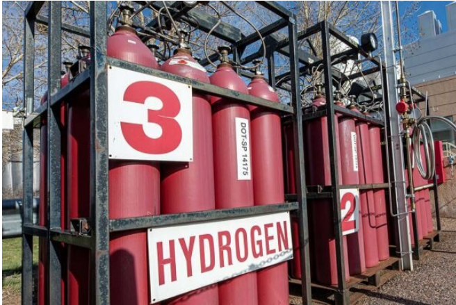
Hydrogen tanks at the National Renewable Energy Laboratory. Credit: Werner Slocum / NREL
